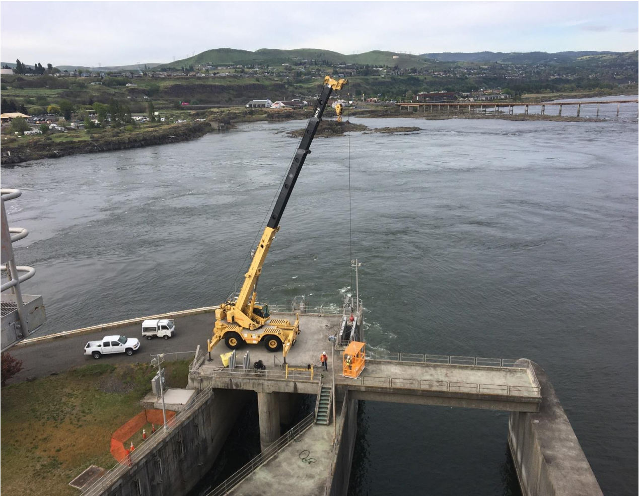
Maintenance setting up to remove loose staff gage sticking out in flow
